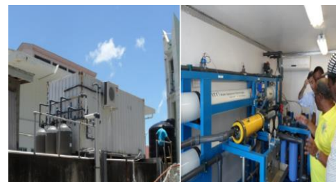
External and Internal View of the Desalination Plant, Bequia
