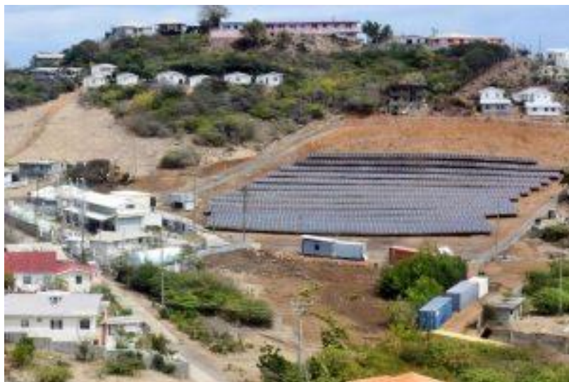
Electricity on Union Island can now be produced using solely solar photovoltaic (PV) and battery energy storage (Searchlight)
