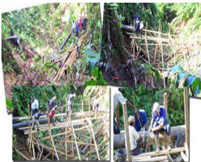
CWSA employees and volunteers repairing water pipes in the Buccament Bay area (The Vincentian)
